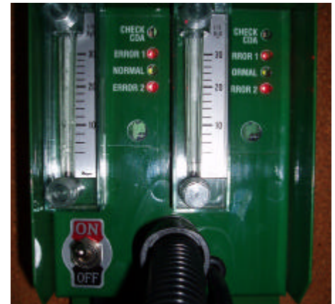
Lights showing on control box
